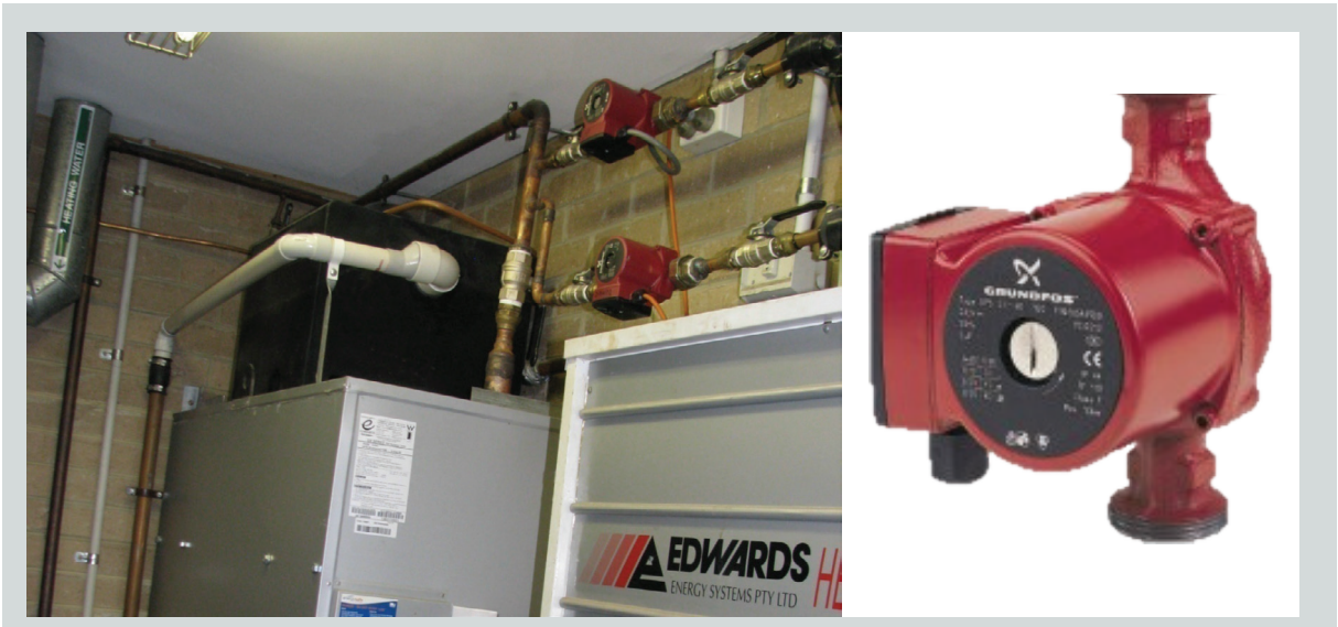
For Small Projects, it is Common to Install a Grundfos Ups 20-60 or Similar to One or Two Circuits. Continuous Flows in Flow and Return Pipes Should Not Exceed a Velocity of 0.5 m/s.
