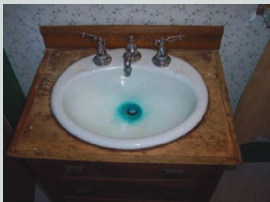
Figure 6.3 Cuprosolvency staining of sanitary ware
