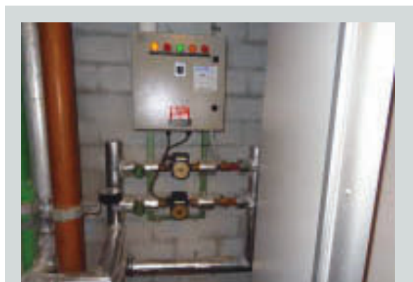
Figure 16.14 Heated Circulating Pumps
