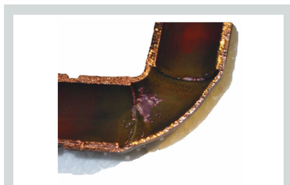
Figure 6.8 Erosion Corrosion from turbulence caused by burr left inside of tube
