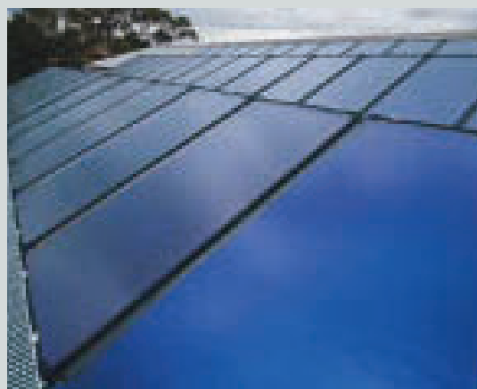
Figure 14.6 Solar panel installation – domestic and commercial
