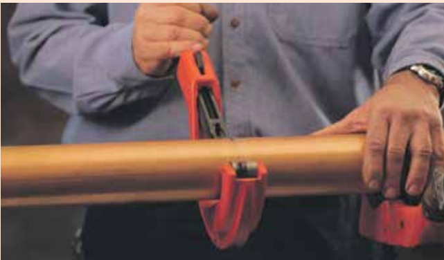
1. Cut copper tube to length using a pipe cutter or fine tooth saw and ensure the pipe is cut square.
