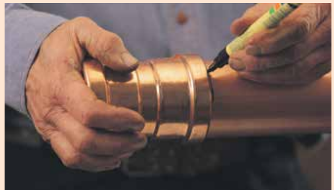
4. Mark the insertion depth on the tube by lining up the fitting side by side with the tube or by inserting the fitting onto the tube until it reaches the tube stop. When fitting is inserted onto the tube the outer edge of the fitting must line up with the marking.
